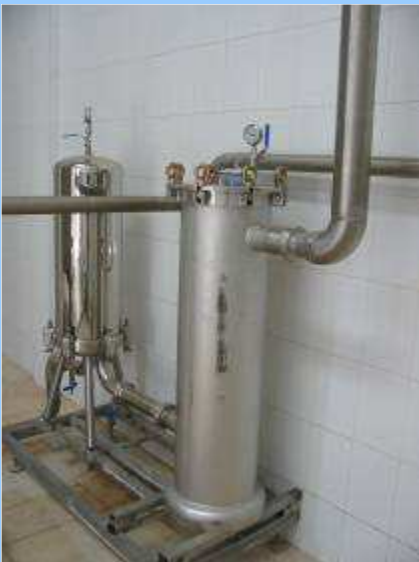
Filtration skid 35 m 3 /h,
