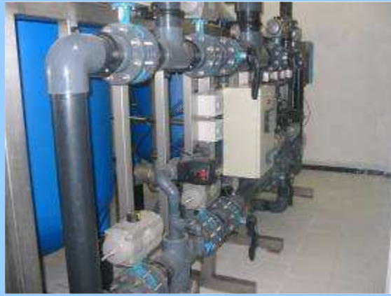
Duplex water softener driven by a set of pneumatic valves and managed by a central electrical panel 50 m 3 /h
