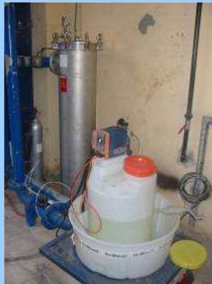
Chlorination before storage
