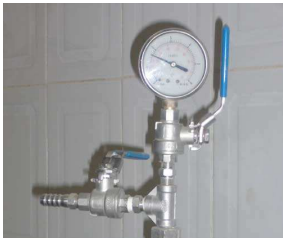
Pressure control system
